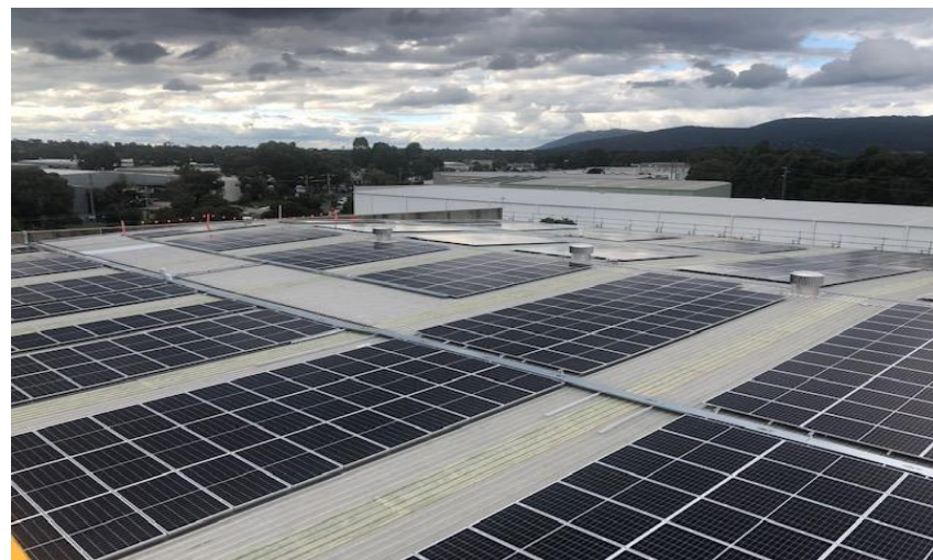
632Kw solar system - 81 Rushdale St, Knoxfield, Victoria
