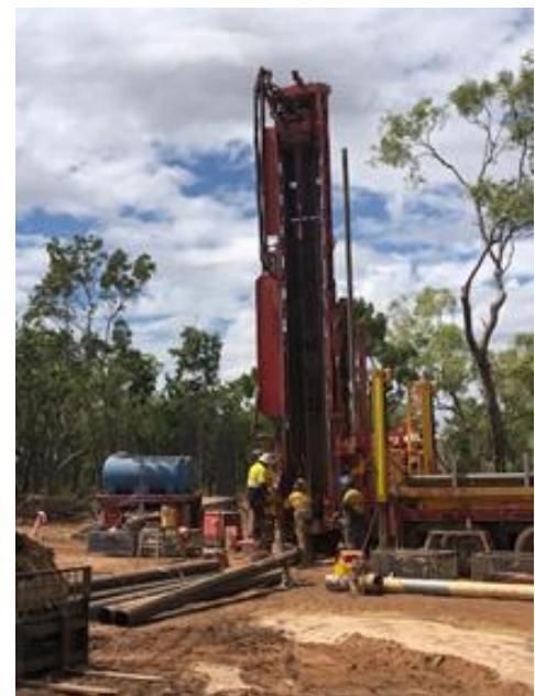
CASING WATER BORE
