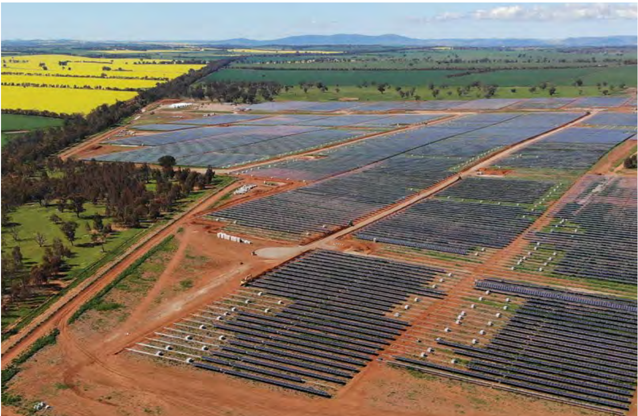
Construction has commenced on the development of a solar farm outside Junee in regional New South Wales. It is one of three solar farms from which Coles will source 10% of its national power needs. The other two solar farms will be located outside the regional centres of Wagga Wagga and Corowa. All three solar farms are being developed and constructed by Metka EGN Australia.
