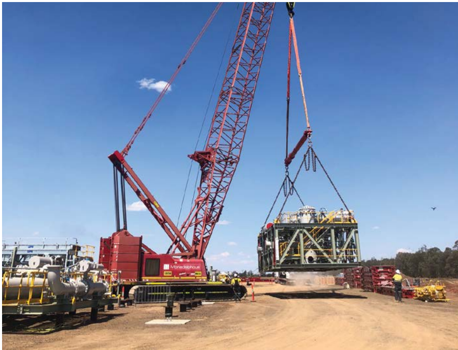
A 250 tonne crawler crane unloading module 153 at Origin's Talinga Orana Gas Gathering Station, Chinchilla, Queensland.
