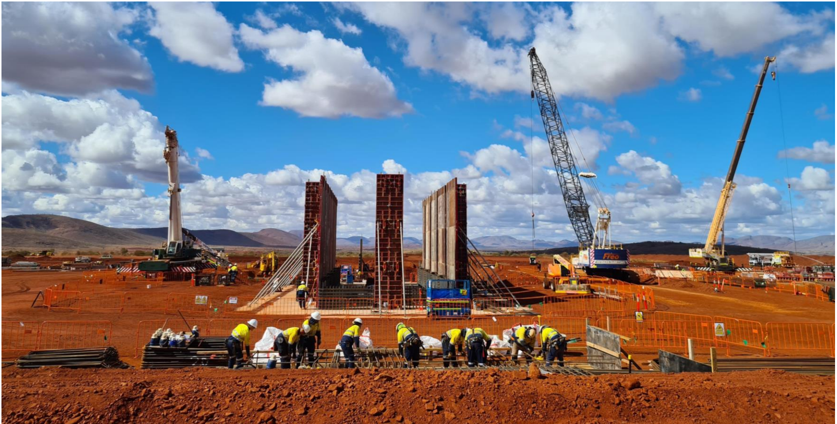
Mondium preparing reinforcing bar for the primary crusher vault at Rio Tinto's Western Turner Syncline Phase 2 mine, Pilbara region, WA.
