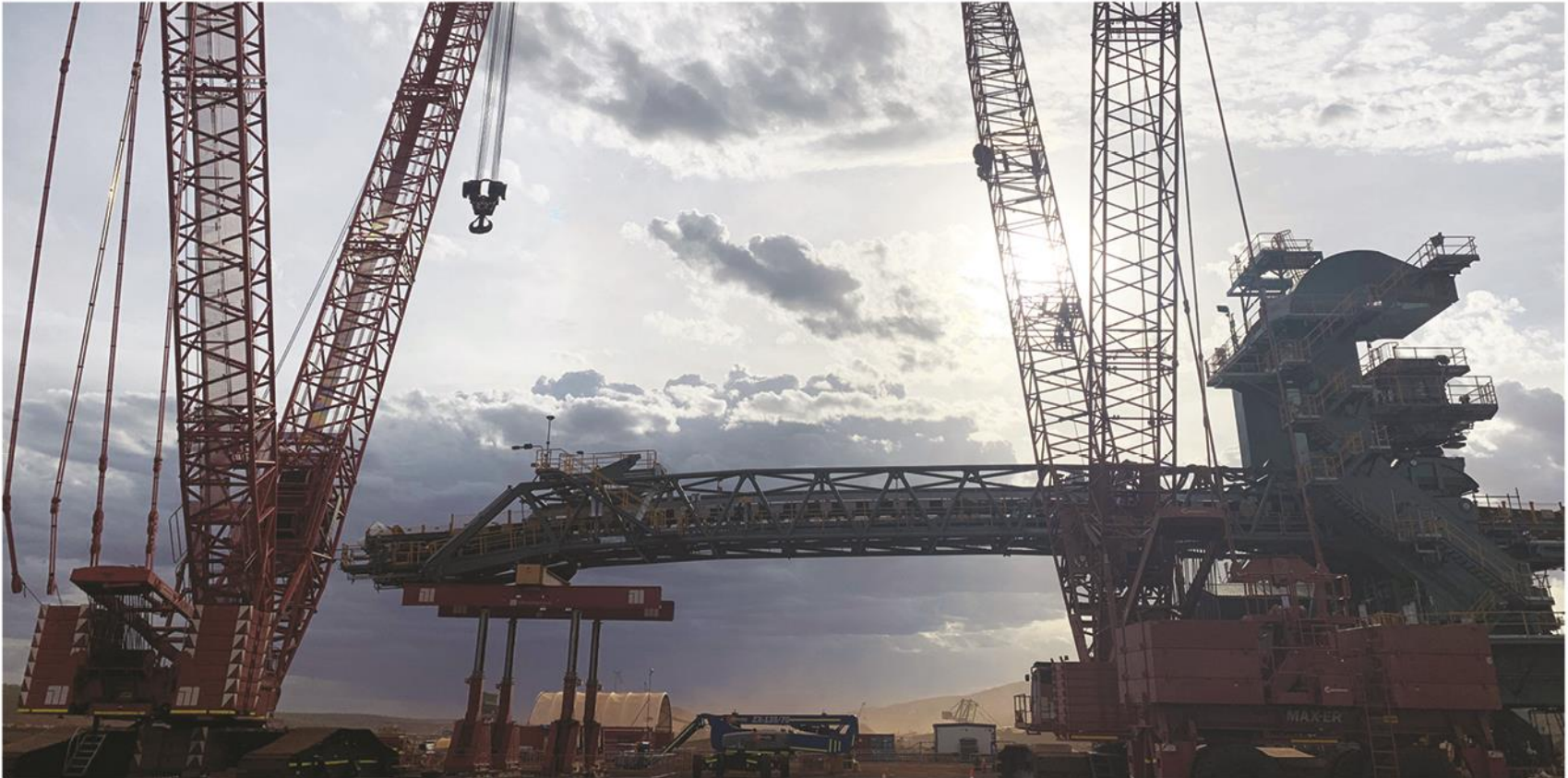
Monadelphous cranes lifting the stacker conveyor boom into final position at BHP's South Flank Project, Newman, WA.
