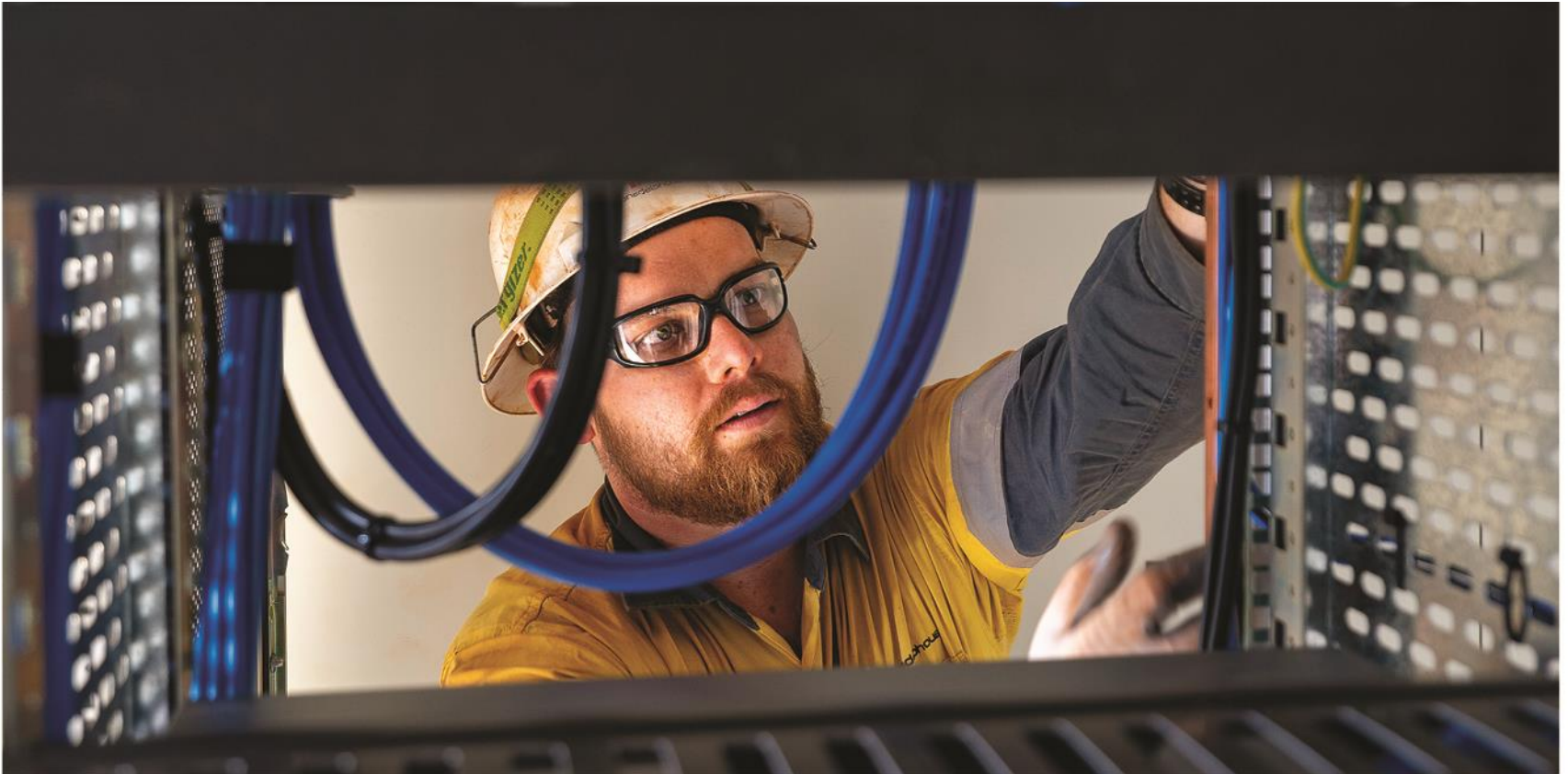
A Monadelphous employee installing equipment in the long-term evolution tower at BHP's Jimblebar, Newman, WA.
