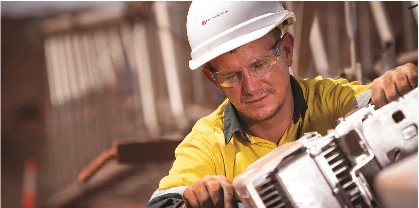
A Monadelphous employee installing equipment in the long-term evolution tower at BHP's Jimblebar, Newman, WA.
