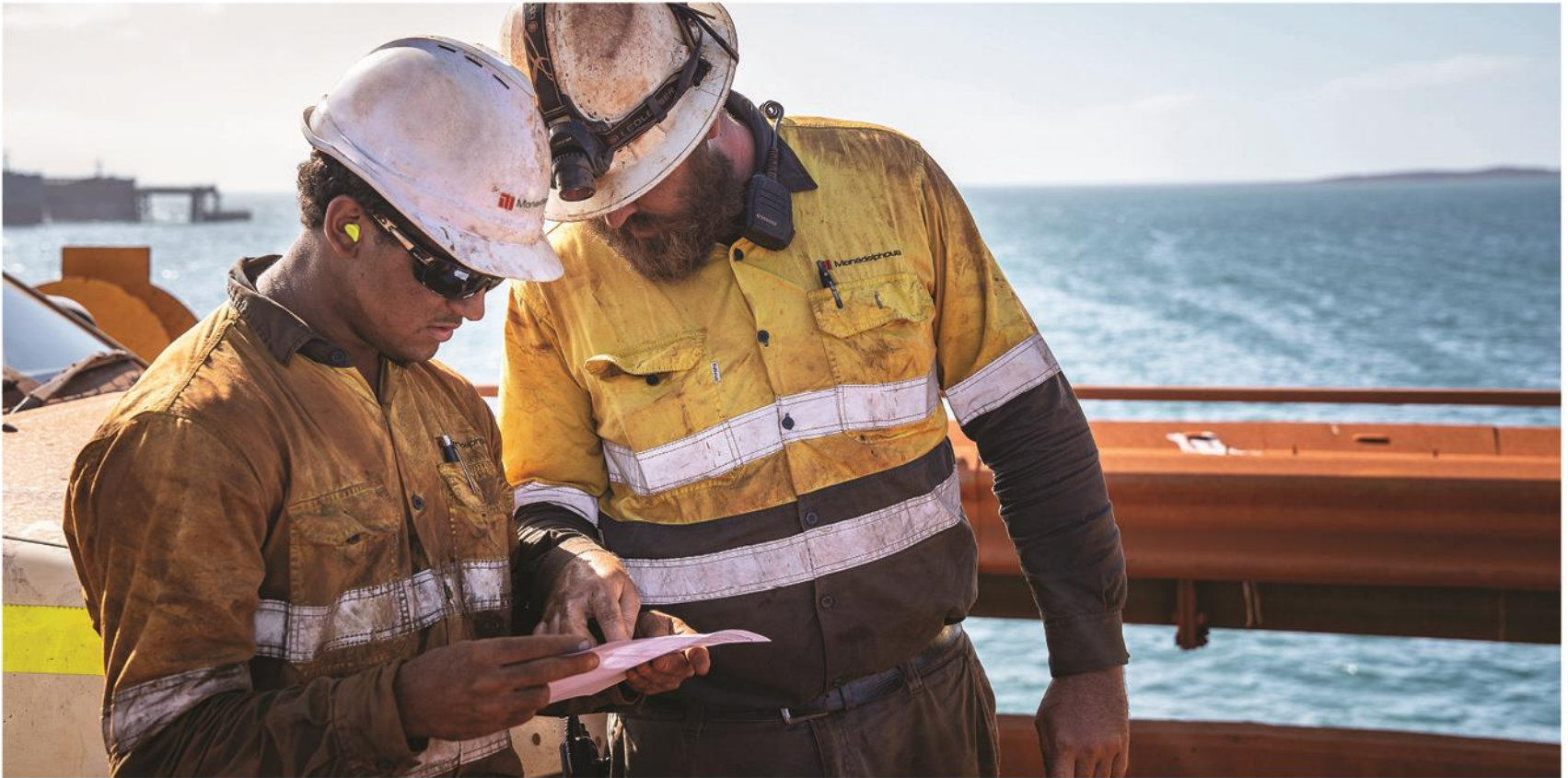
Monadelphous employees preparing for idler changeout at Cape Lambert, Pilbara region, WA.
