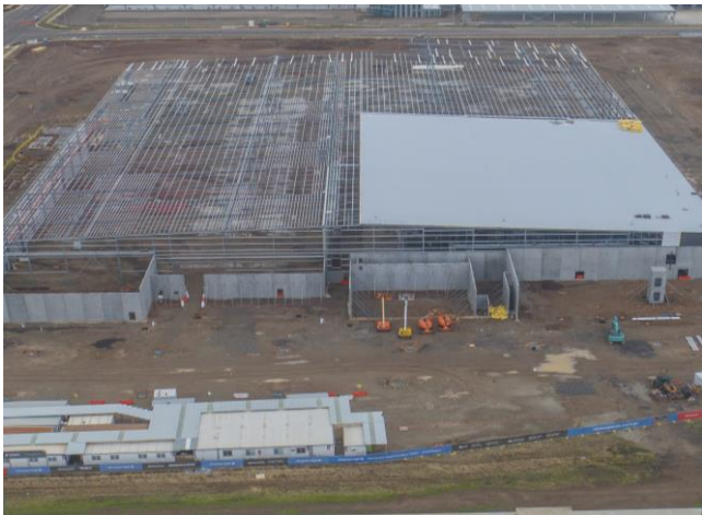
Construction at the Melbourne Ocado online customer fulfilment centre progressed during the half.
