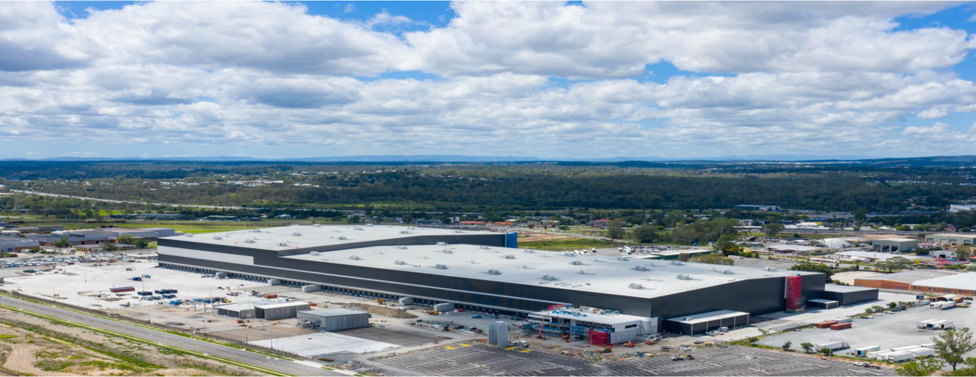
Construction at the Queensland Witron automated distribution centre progressed during the half.
