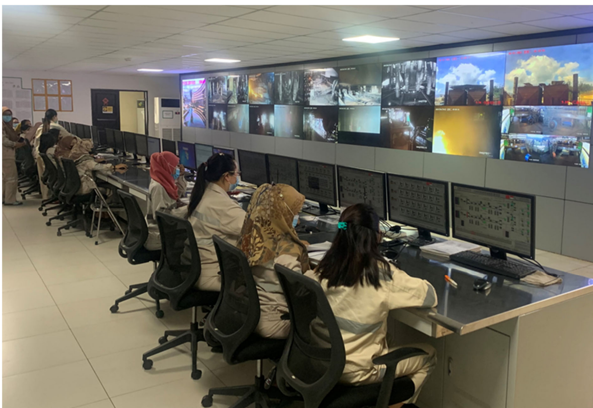
Hengjaya Nickel control centre
