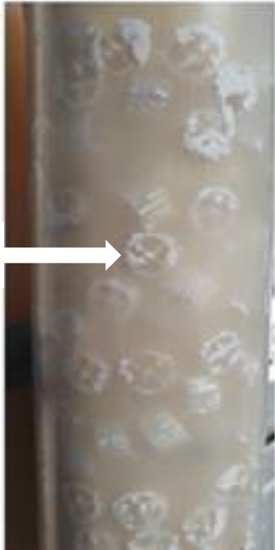
Fouling of absorber packing with unfiltered solution
