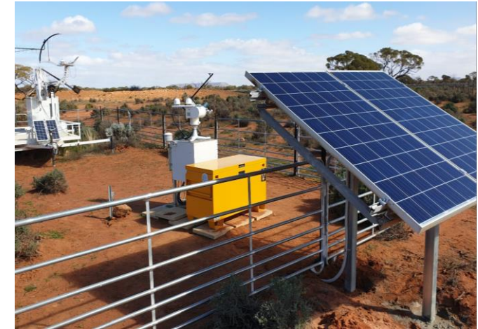
Solar monitoring station on-site
