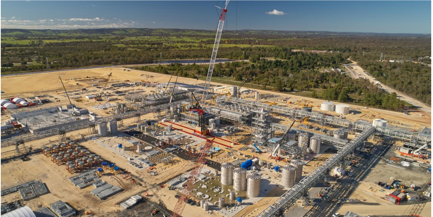
Construction underway at the MARBL Lithium Joint Venture's Kemerton Plant, south-west region, WA.
