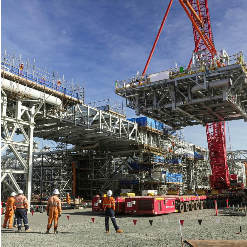
Heat exchanger module being lifted into position at the Woodside-operated Pluto LNG Plant, Karratha, WA.
