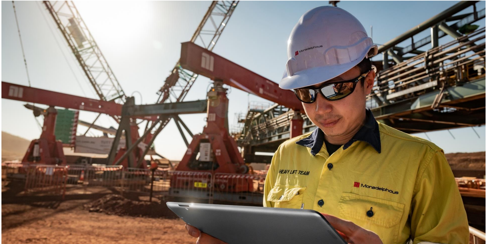
A Monadelphous employee reviewing engineering plans for a major lift at BHP's South Flank Project, Pilbara, WA.
