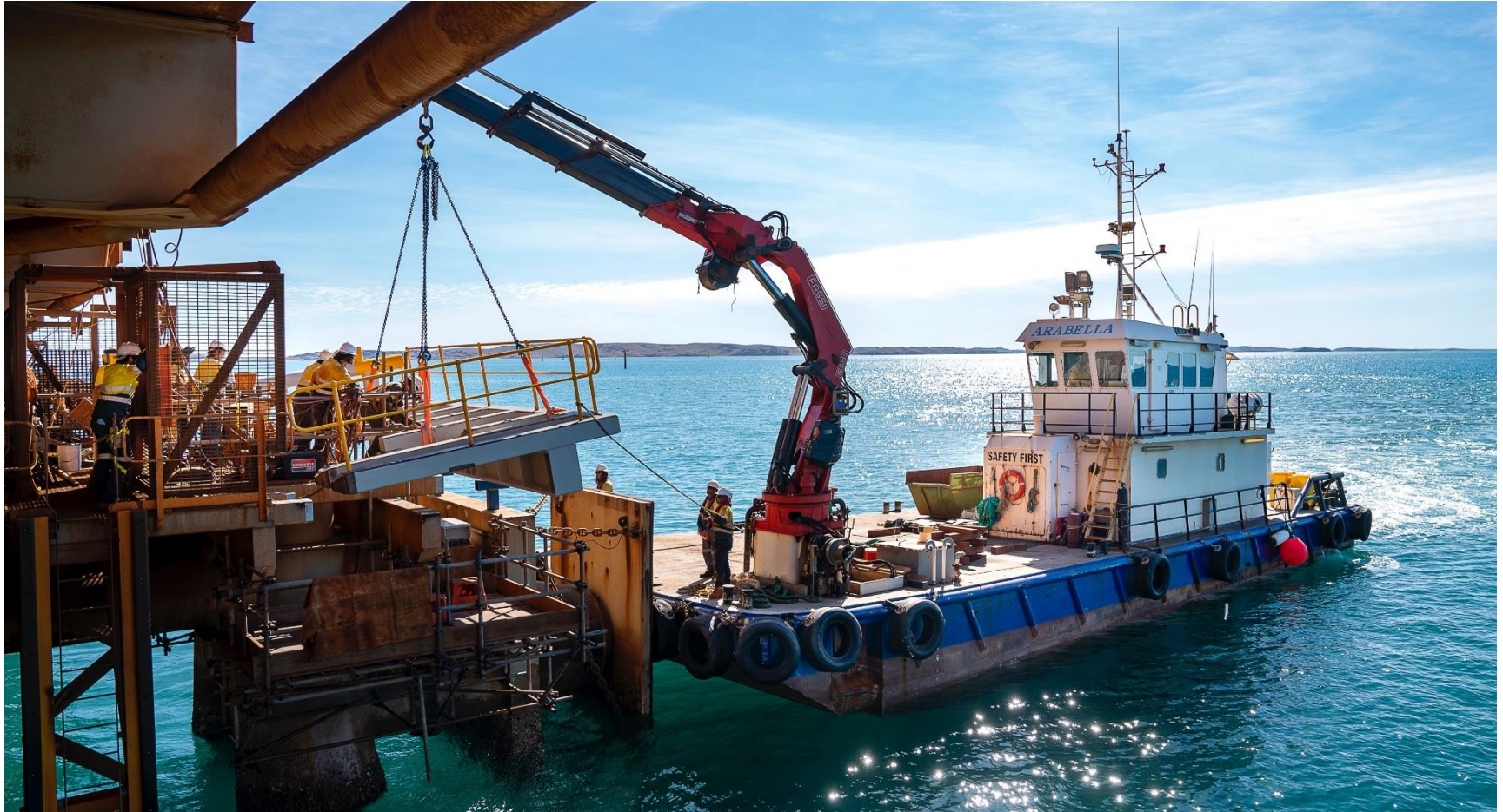
Sustaining capital projects work being undertaken at Parker Point near Dampier, WA.
