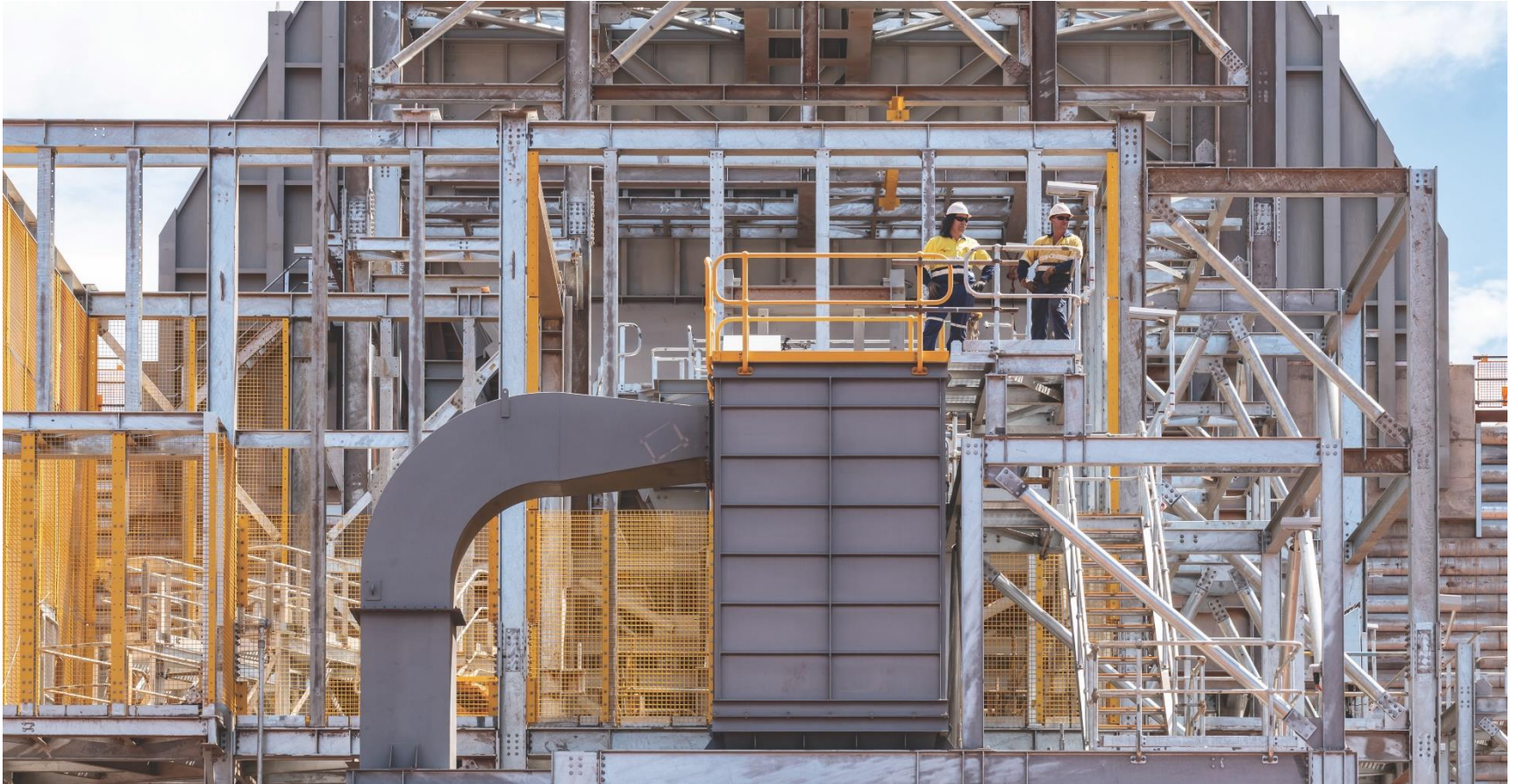
Monadelphous employees on the newly constructed primary crusher at Rio Tinto's West Angelas Deposits C & D Project, Newman, WA.
