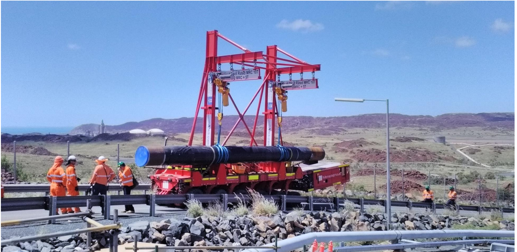
Monadelphous' self-propelled modular transporter Davit frame in operation at the Woodside-operated Pluto LNG Plant, Karratha, WA.
