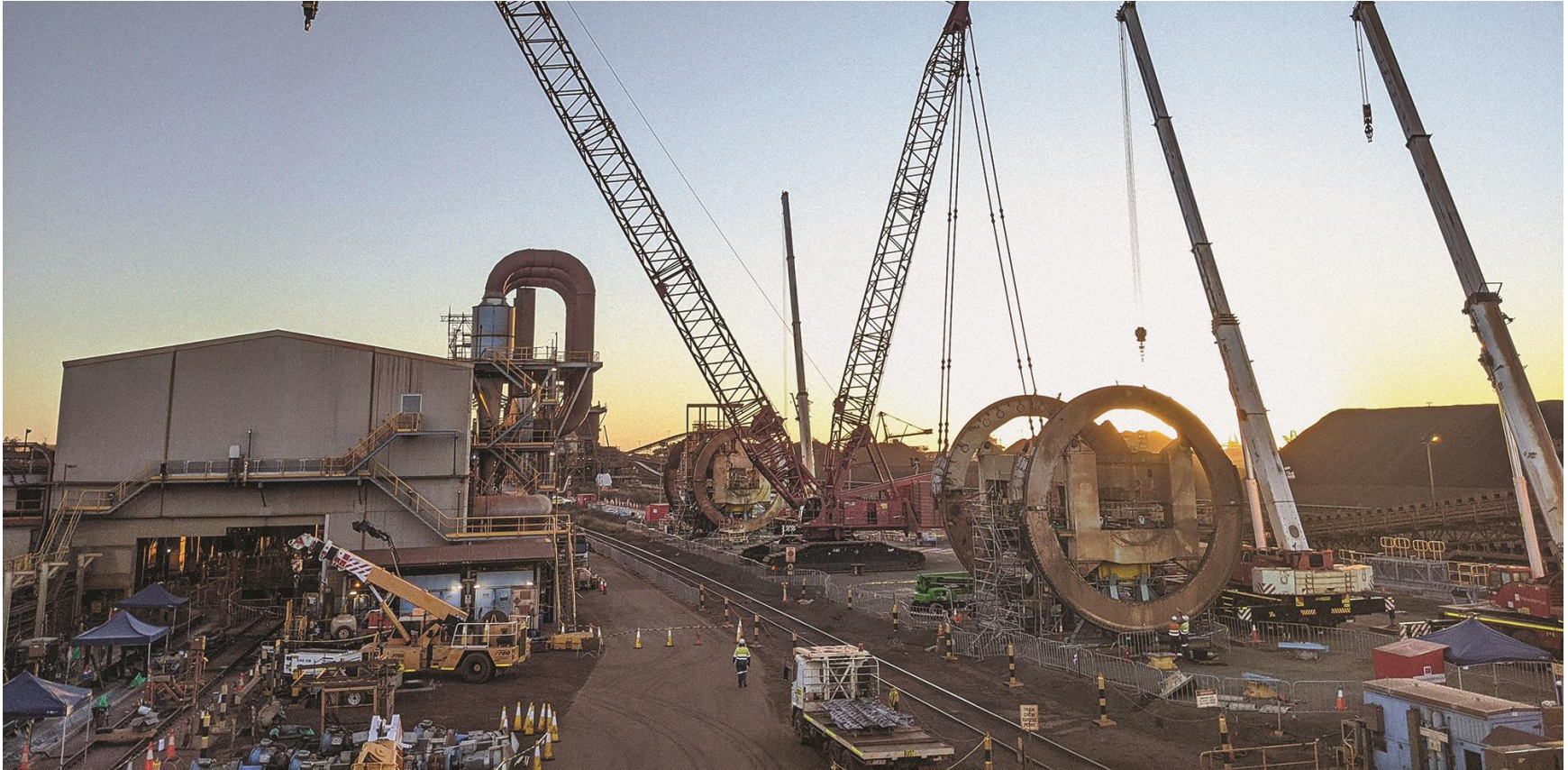
Car dumper refurbishment work undertaken by Monadelphous at BHP's Nelson Point Operations, Port Hedland, WA.
