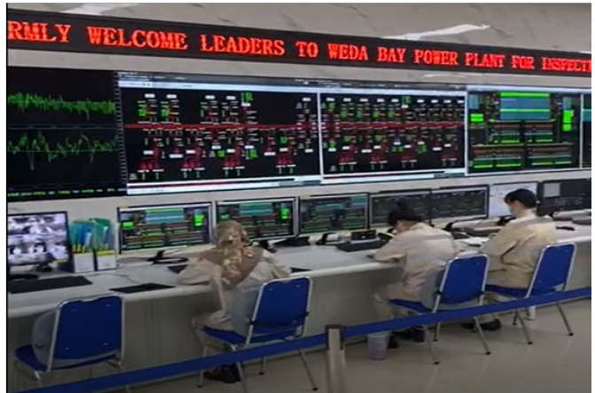
Weda Bay Power Plant control room
