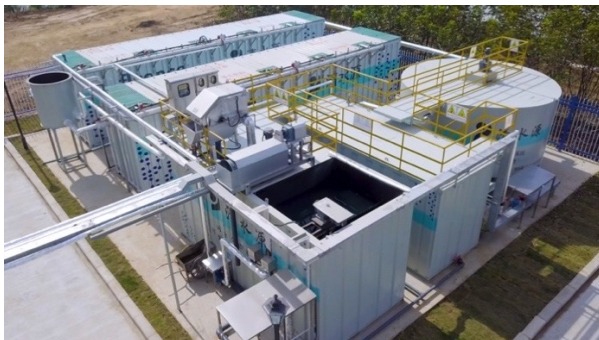
Rural Aspiral plant, Luoyang, Henan province
