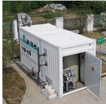
Aspiral S1 near homes, Hefei, Anhui province
