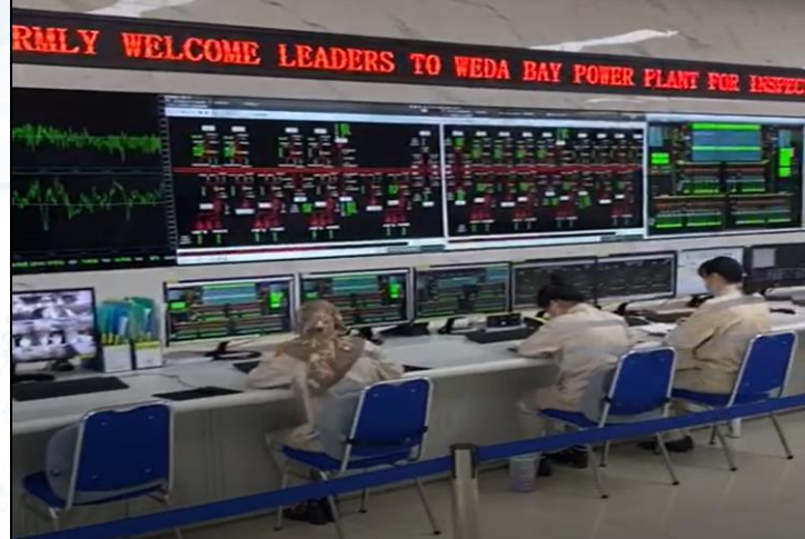
Weda Bay Power Plant control room
