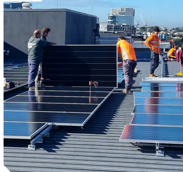
Solar panel installation was completed at 52 Merivale Street, South Brisbane, QLD in June 2022
