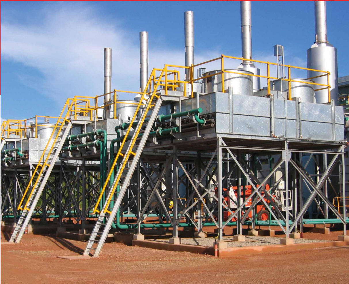
Power generation station at Wiepa, QLD. Air Radiators Industrial (Gillman, SA) provided cooling for 6 x 4.5MW diesel generators.
