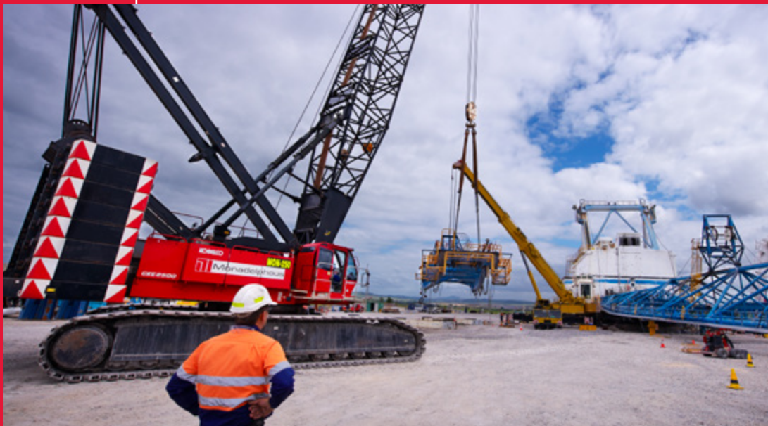
A Monadelphous crawler crane being used in the 2000s to complete work on a dragline at Rio Tinto Coal Australia's Hunter Valley Operations, which has since been sold by Rio Tinto.
