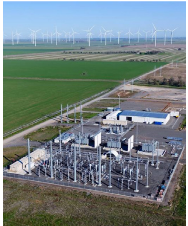
Murra Warra Stage II Wind Farm, located in regional Victoria, comprising 38 wind turbines with a capacity of 209MW.
