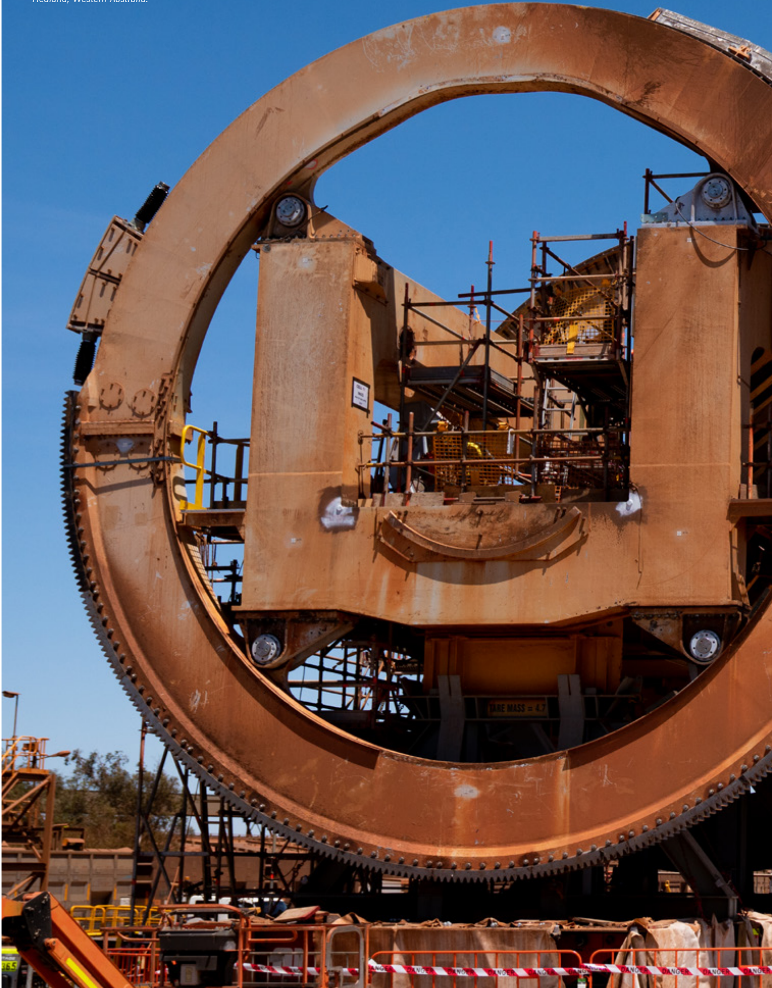
Monadelphous undertaking Car Dumper 1 Mega Shut at BHP's Nelson Point, Port Hedland, Western Australia.
