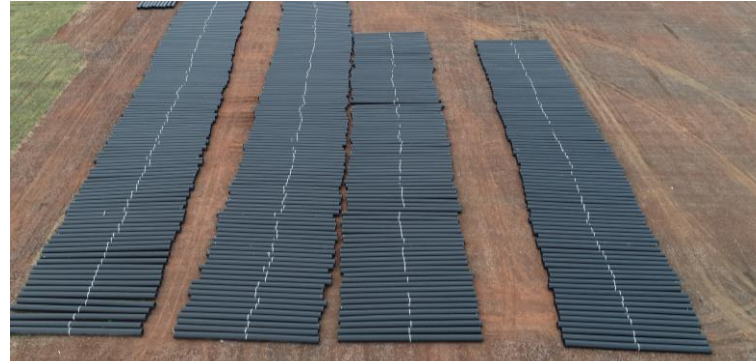
Pipes for irrigation pipeline to total 6 kms from Fitzroy River to Rookwood Farms (September 2022).
