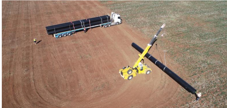
Delivery of 20 m long, 1 m diameter poly pipes for irrigation at Riverton (July 2022).
