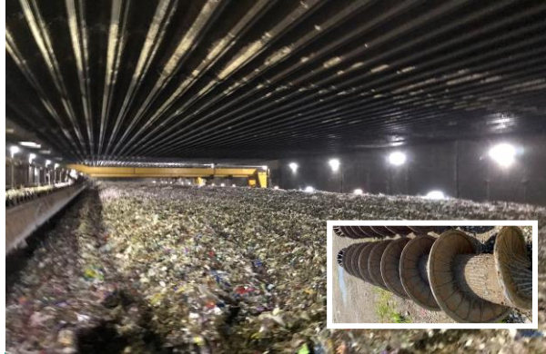
Composting hall at GRL with auger inset
