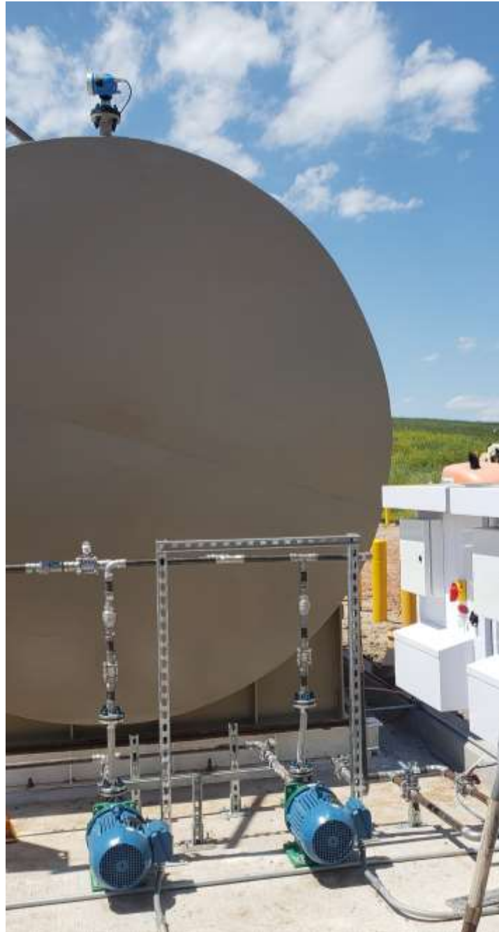
Figure 3: Bulk Storage Acid Tank and Pumps
