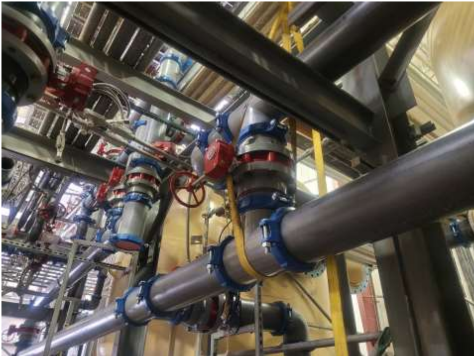
Figure 2: Updated plumbing on Ion Exchange Column
