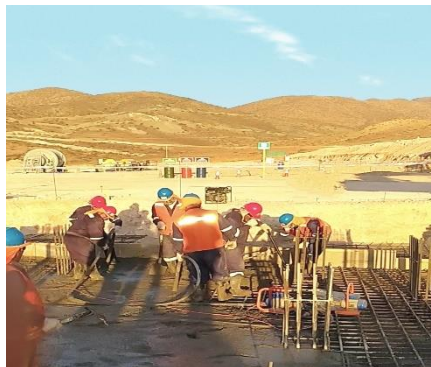
The Mariposa team laying the foundations in preparation for the Installation Phase
