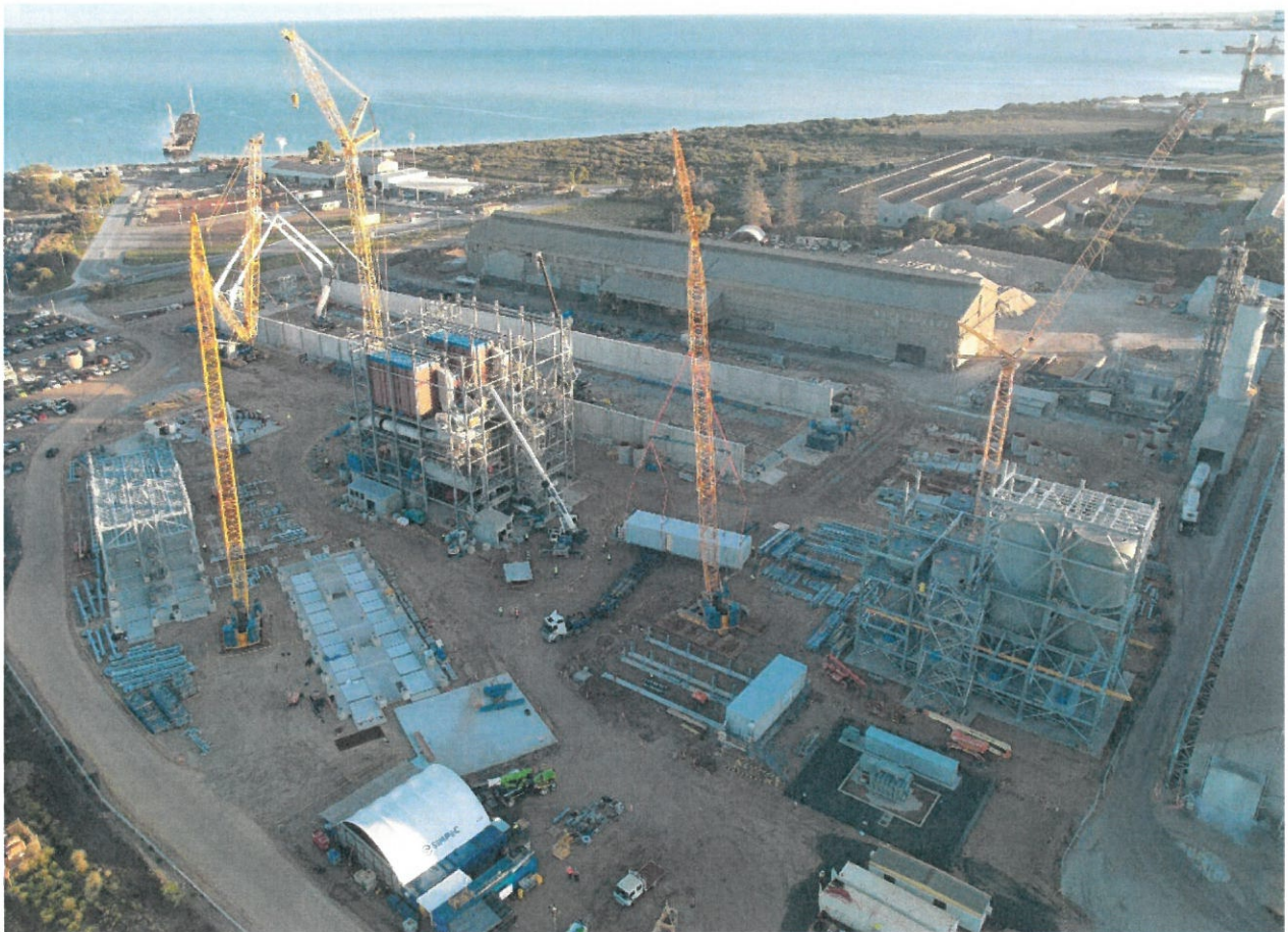
Current Progress photo of Kwinana Cockburn Cement upgrade – performed by SIMPEC under a LNTP.
