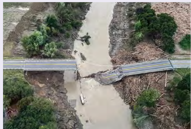
Damage to the regional fibre route on the bridge crossing the Hikuwai River, north of Gisborne, required 800 metres of fibre to be overlaid.
