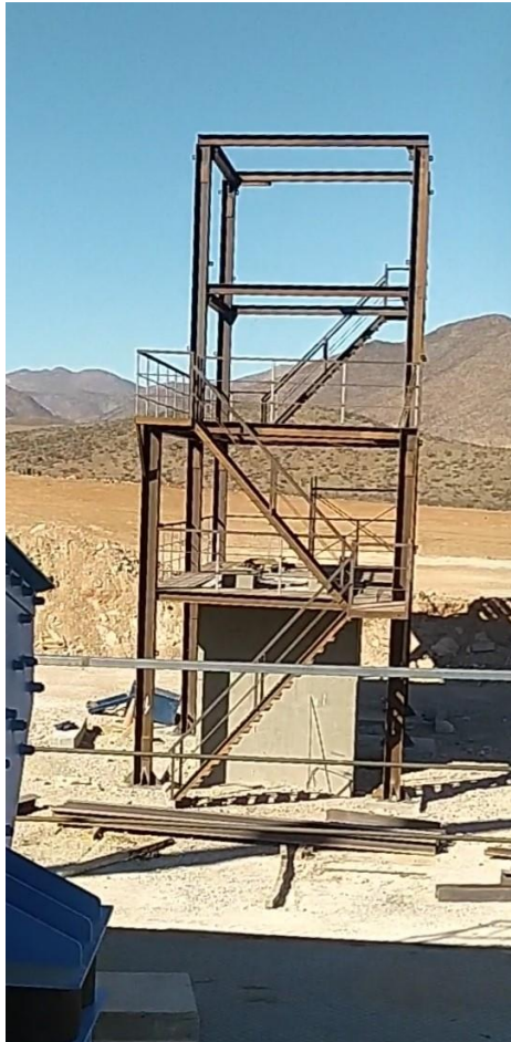
Figure 2: Fine crushing platform
