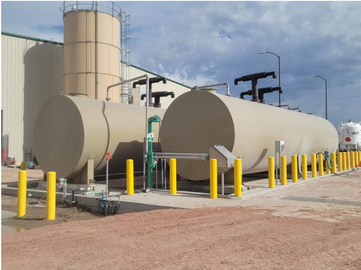
Figure 5: Bulk sulphuric acid storage facilities at Lance
