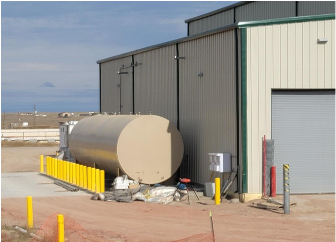
Figure 6: Installed high-capacity hydrogen peroxide storage tank
