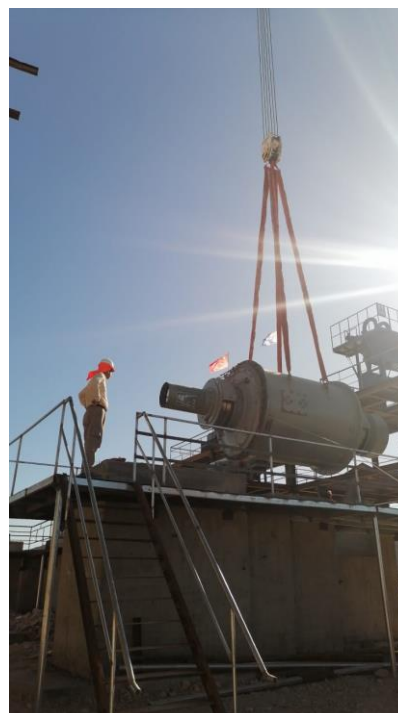
Figure 2: Ball mill on operating platform
