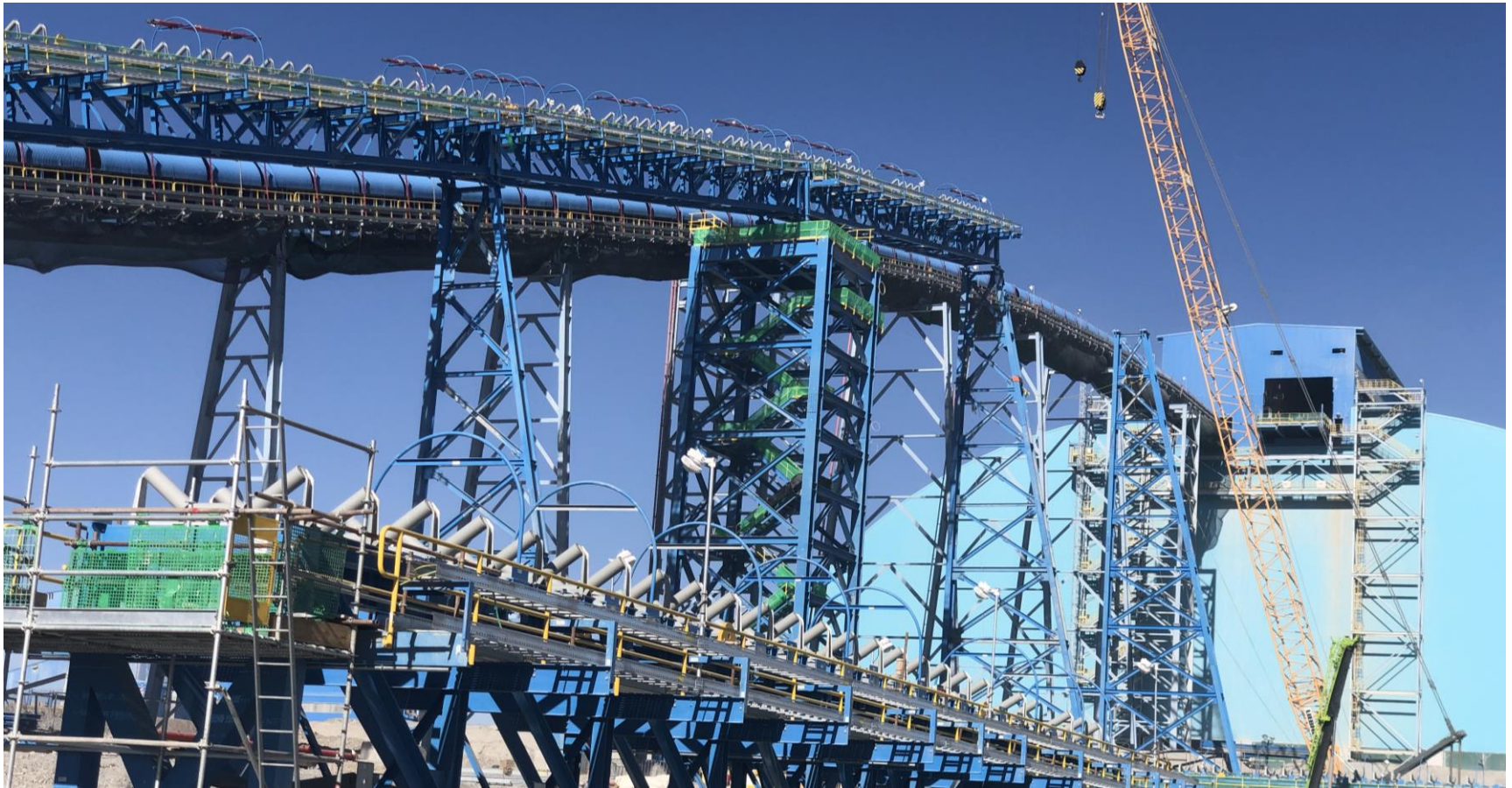
An overland conveyor at Oyu Tolgoi Underground Project, Mongolia.
