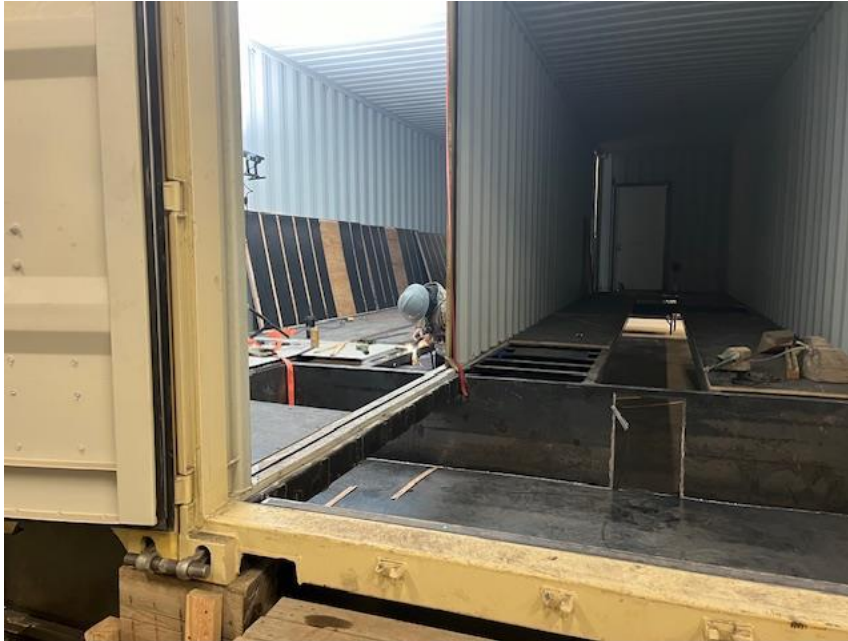
Figure 3 - Header House #11 under construction. MU-3 and beyond header houses will accommodate twice the number of wells as previous header houses
