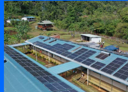
Solar mini-grid, Pimaga Rural Hospital
