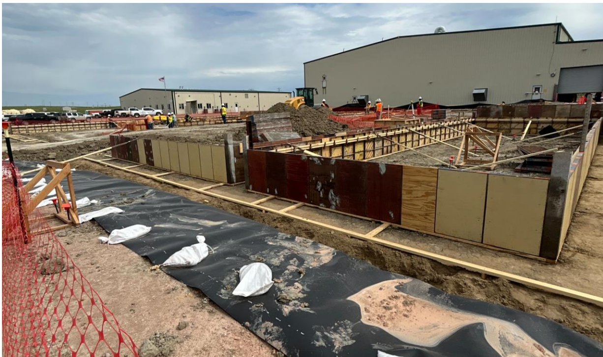
Figure 2: Crews installing forms in preparation for upcoming concrete pours at Ross CPP site
