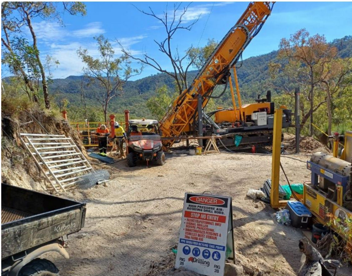
Figure 4. View looking towards the northwest, with the rig drilling hole 24BRD0026 towards the southwest.
