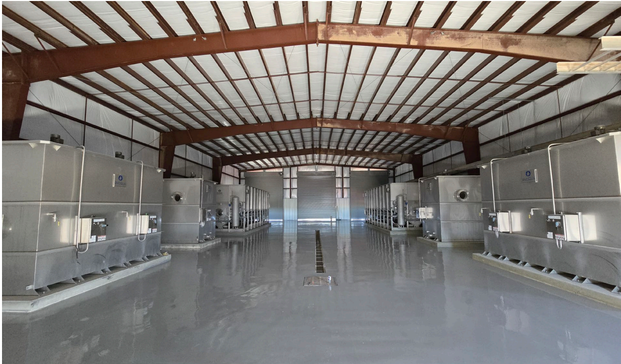
Figure 4: Interior of the new fine solids removal building with major equipment placed
