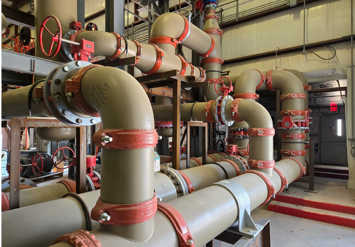
Figure 1: Modified/Upgraded piping systems inside the Ross Satellite Plant
