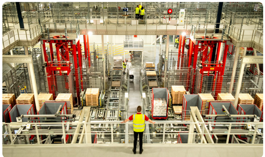
Pictured: Coles has opened its second ADC using global leading Witron technology as part of its more than $1 billion investment in technology led innovation. The site spans 187,000 square metres which is the equivalent size of around 25 rugby league fields.
