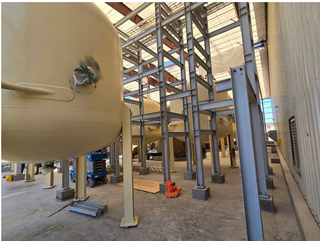
Figure 3: Ion exchange columns and pipe racks placed in new section of plant
