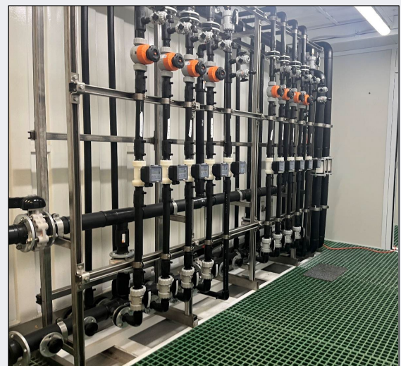
Wellhouse Module (pipe room)
