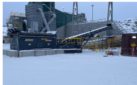
Picture 2: Temporary feeder system
