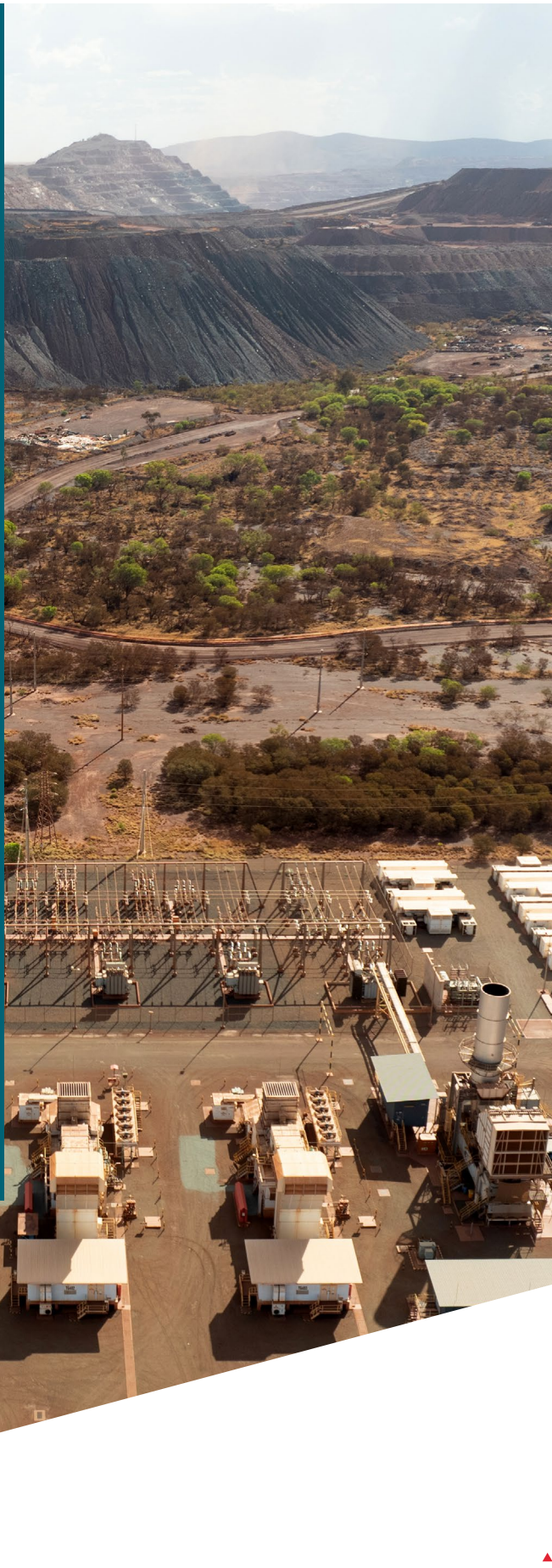
Newman Power Station, WA ▲
