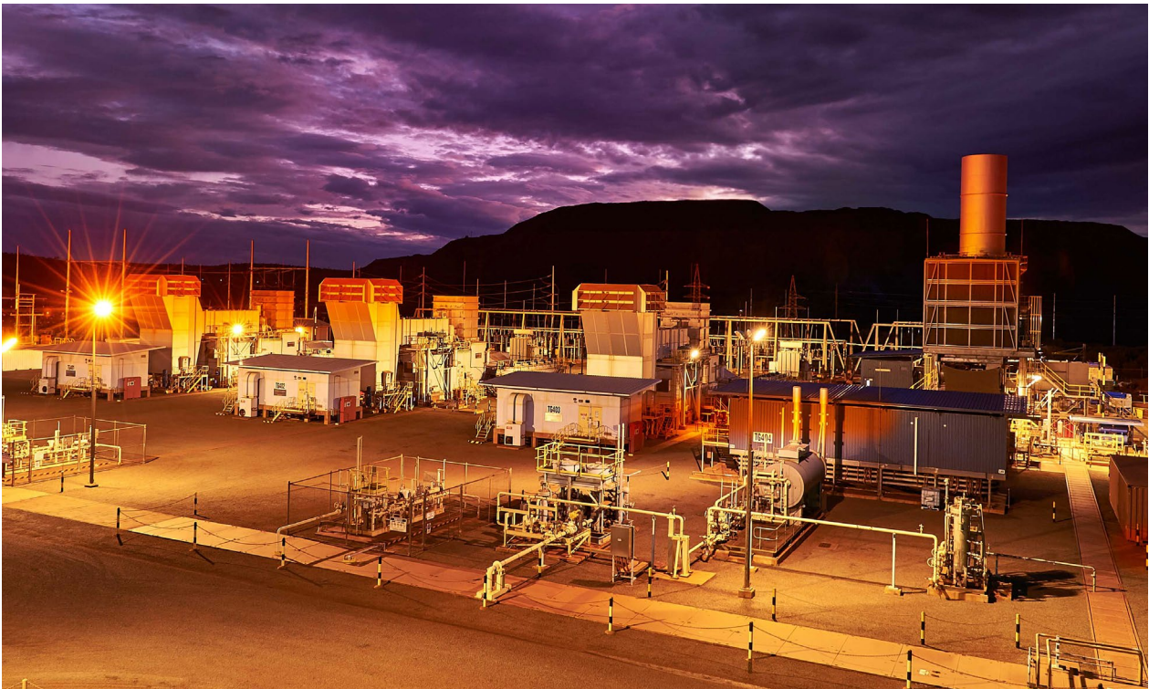
▲ Newman Power Station, WA
