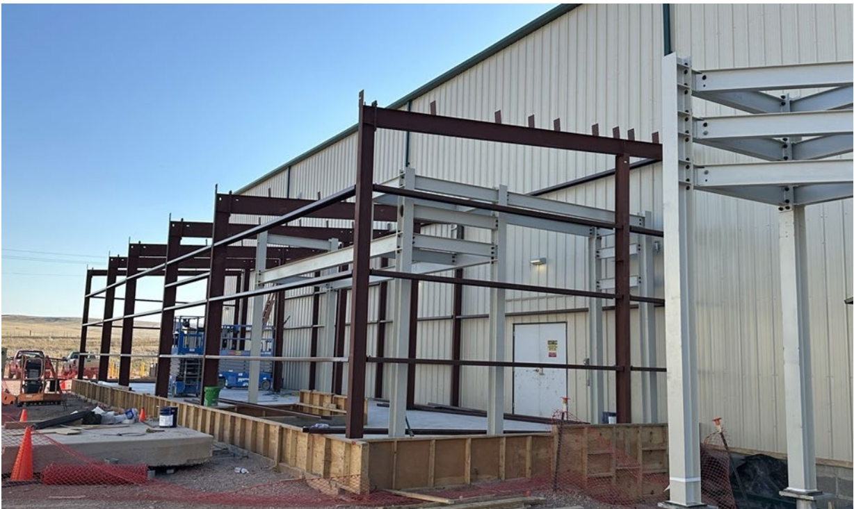
Figure 3: Progress photo of new laboratory addition to the East side of the existing Lance Plant facility
