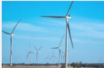
Warradarge Wind Farm
