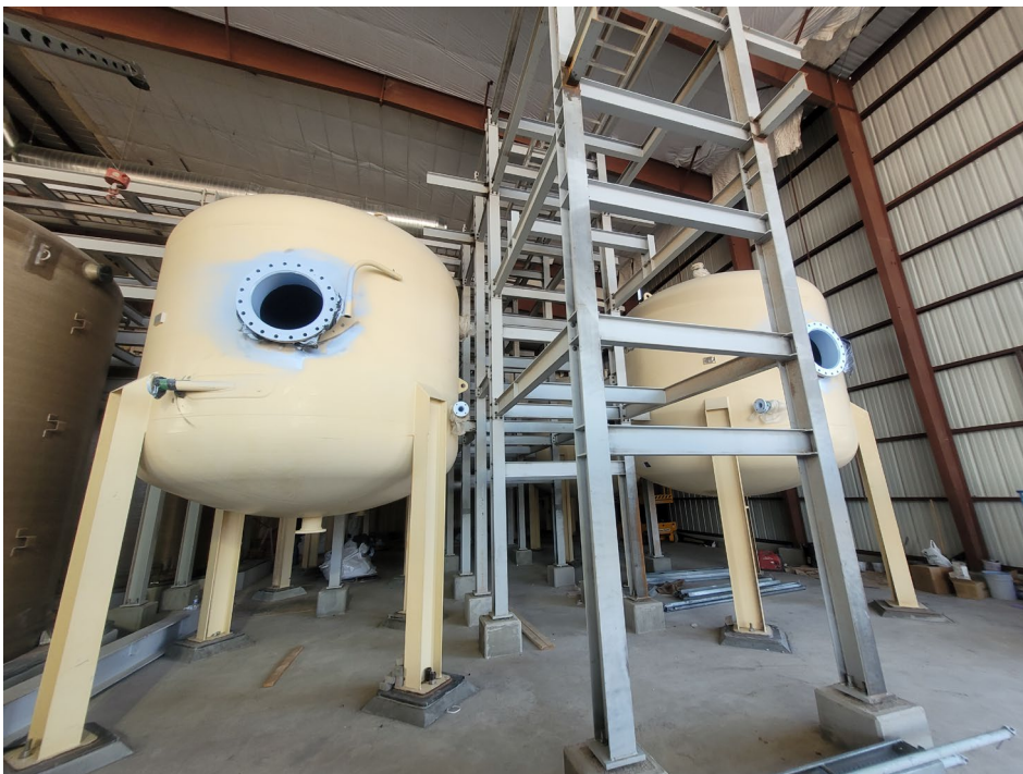
Figure 4: Ion exchange columns and pipe racks in new section of plant
