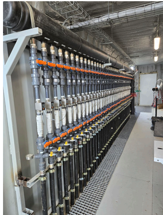
Figure 6: HH-11 interior, production well meter runs
