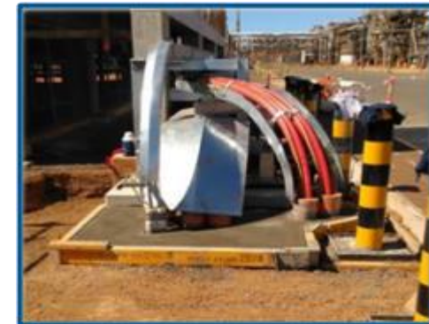
Design-out (operating): Pluto Solar
