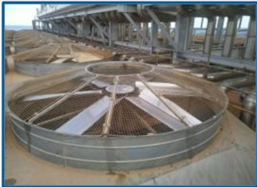
Efficiency: Train 1 fin fans upgrade
