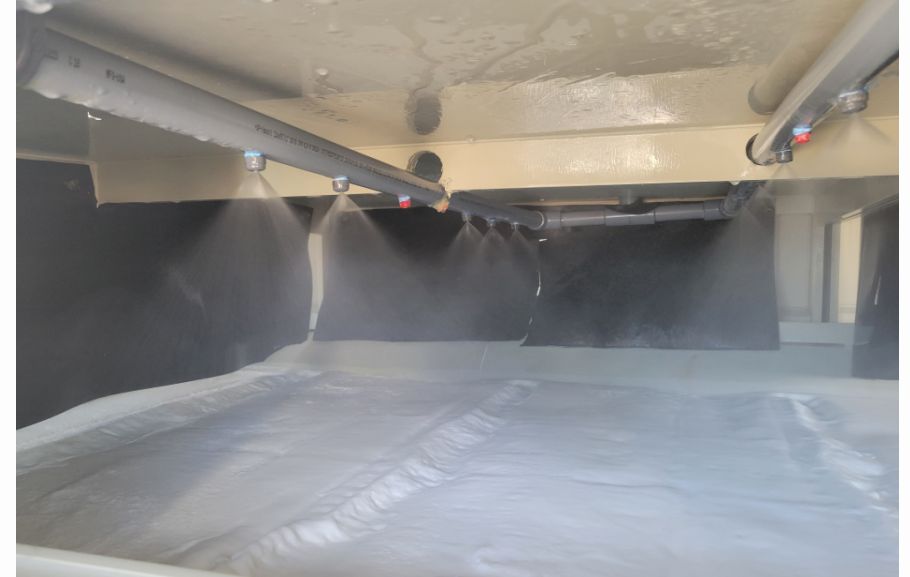
New acid spray bar and nozzles in belt wash area
