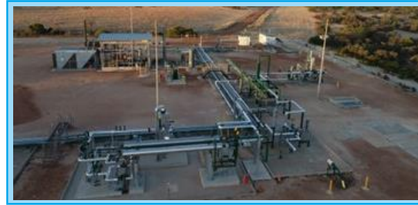
Xyris Gas Plant
