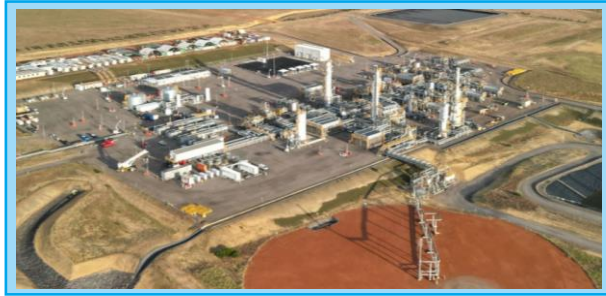
Waitsia Gas Plant
