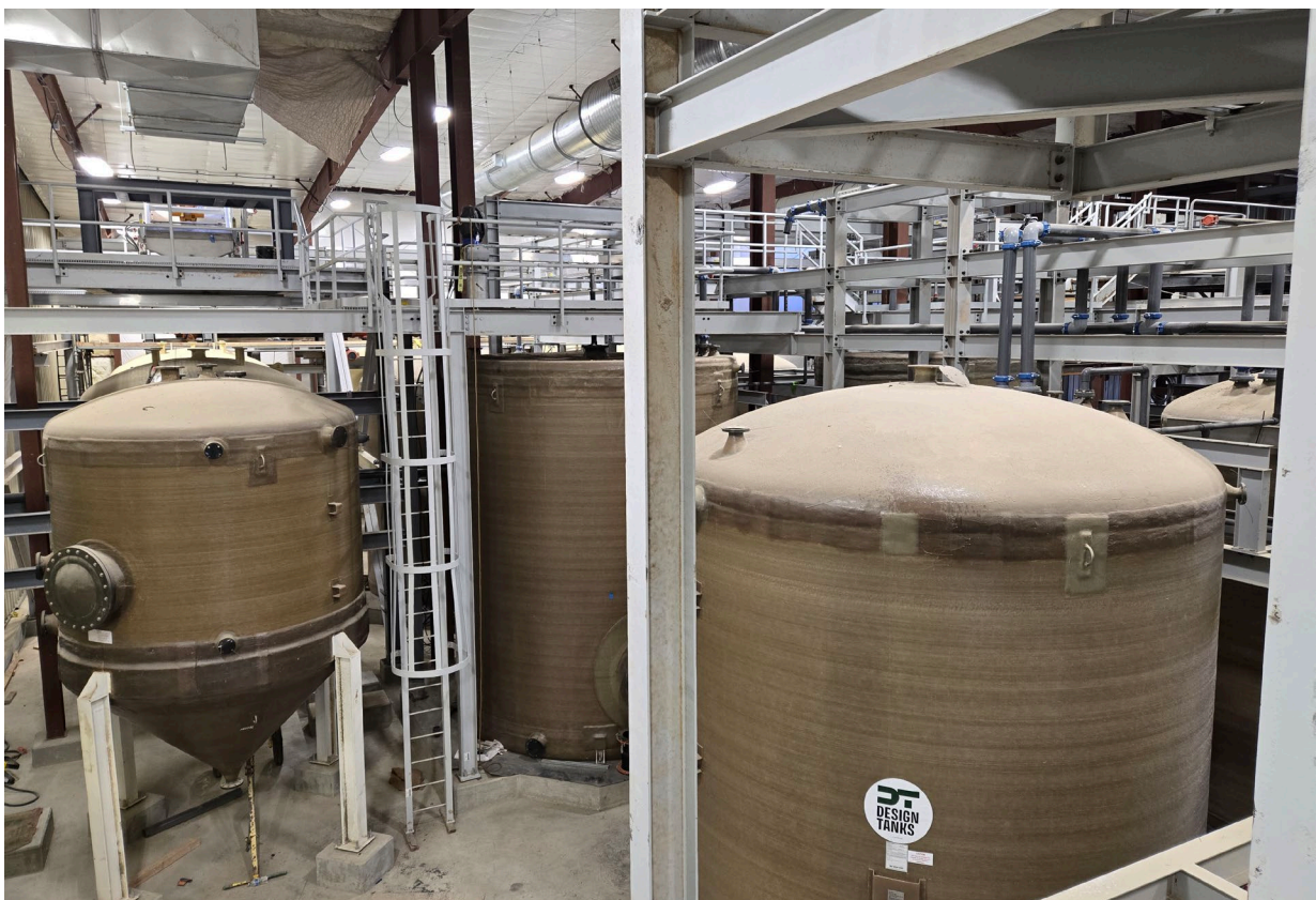
Figure 2: Interior photo of the Lance Central Processing Plant, December 2024
