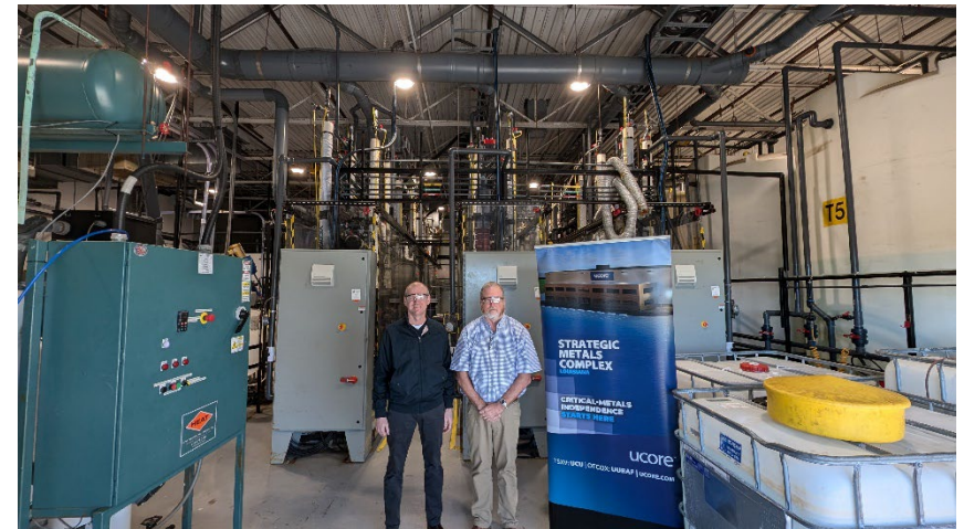
Ucore Rapid SX demonstration plant in Kingston, Canada
