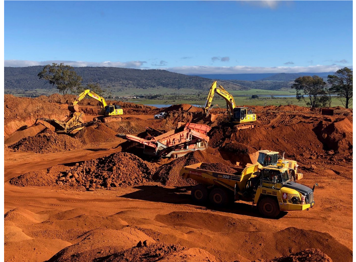
ABx bauxite mining at Bald Hill Project near Campbell Town, Tasmania in 2020
