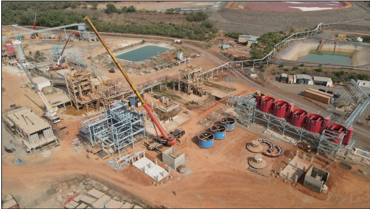
Figure 1: Ball mill and flotation areas in December under construction. The flotation circuit is now 50% complete, while the ball mill areas is 30% complete
