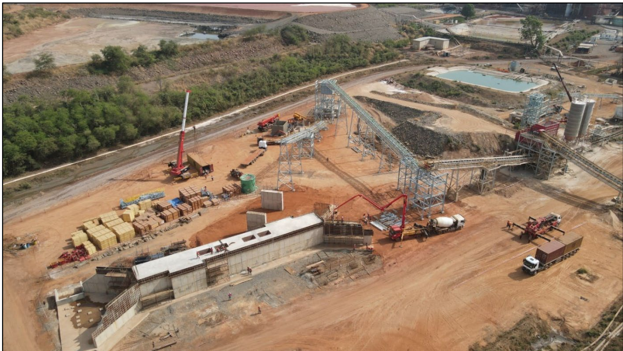
Figure 2: Secondary crusher and sulphide stockpile feed conveyor areas are 35% and 10% complete respectively
