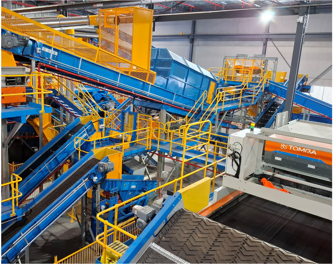
Newly installed Western Sydney Material Recovery Facility processing line in New South Wales
