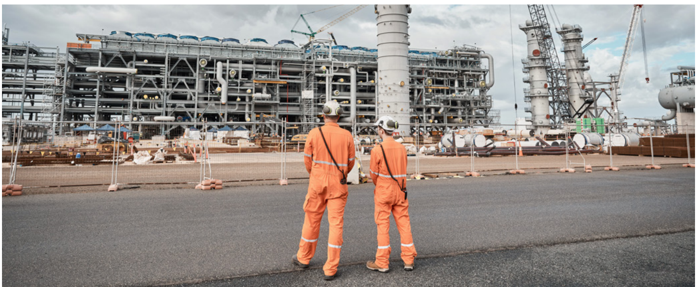
The safe startup of Pluto LNG in 2012 cemented Woodside's status as a major supplier of energy to the Asia-Pacific region. Now, we're developing a second train to process gas from the offshore Scarborough field
