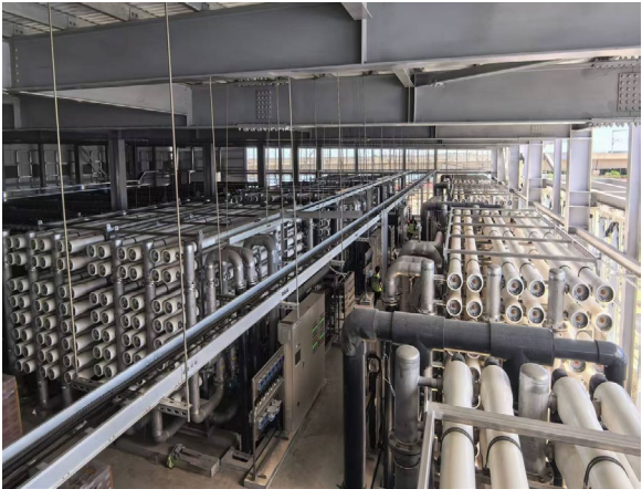
Reverse Osmosis Installed
