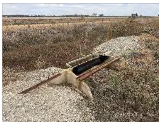
Flood Irrigation Gate
