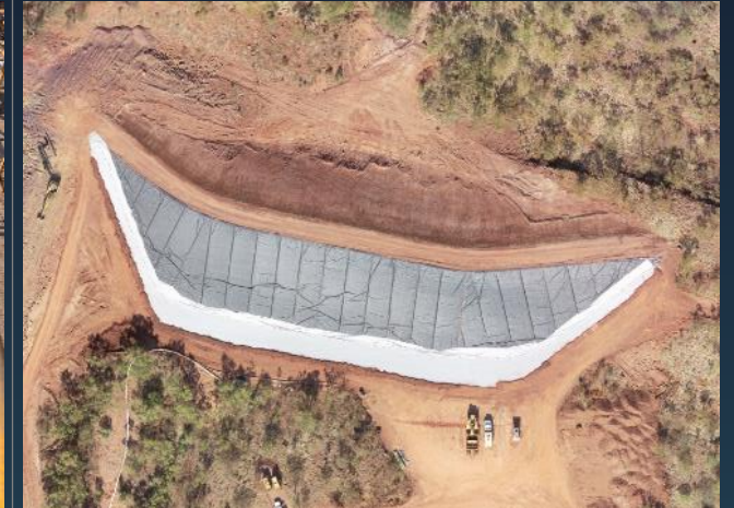
Enhanced water diversion infrastructure
